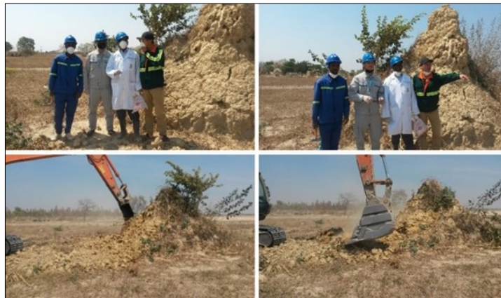
Fig.6. Termite mounds before leveling them and their demolition in action at the site
