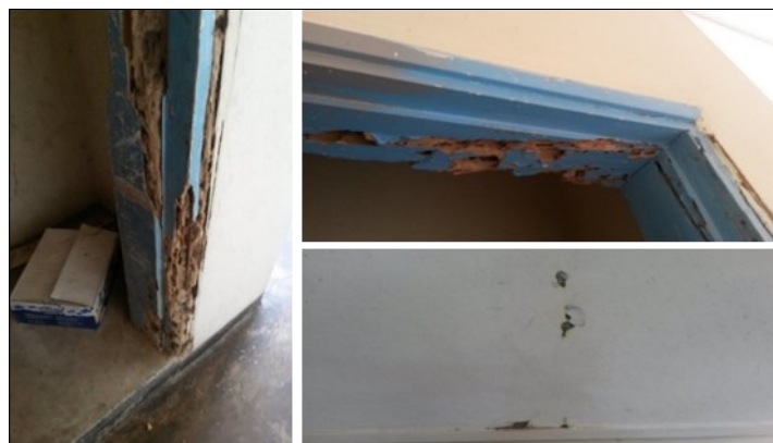
Fig. 16. Termite damage spotted on door frames and boards at CBU offices in Kitwe, Zambia
